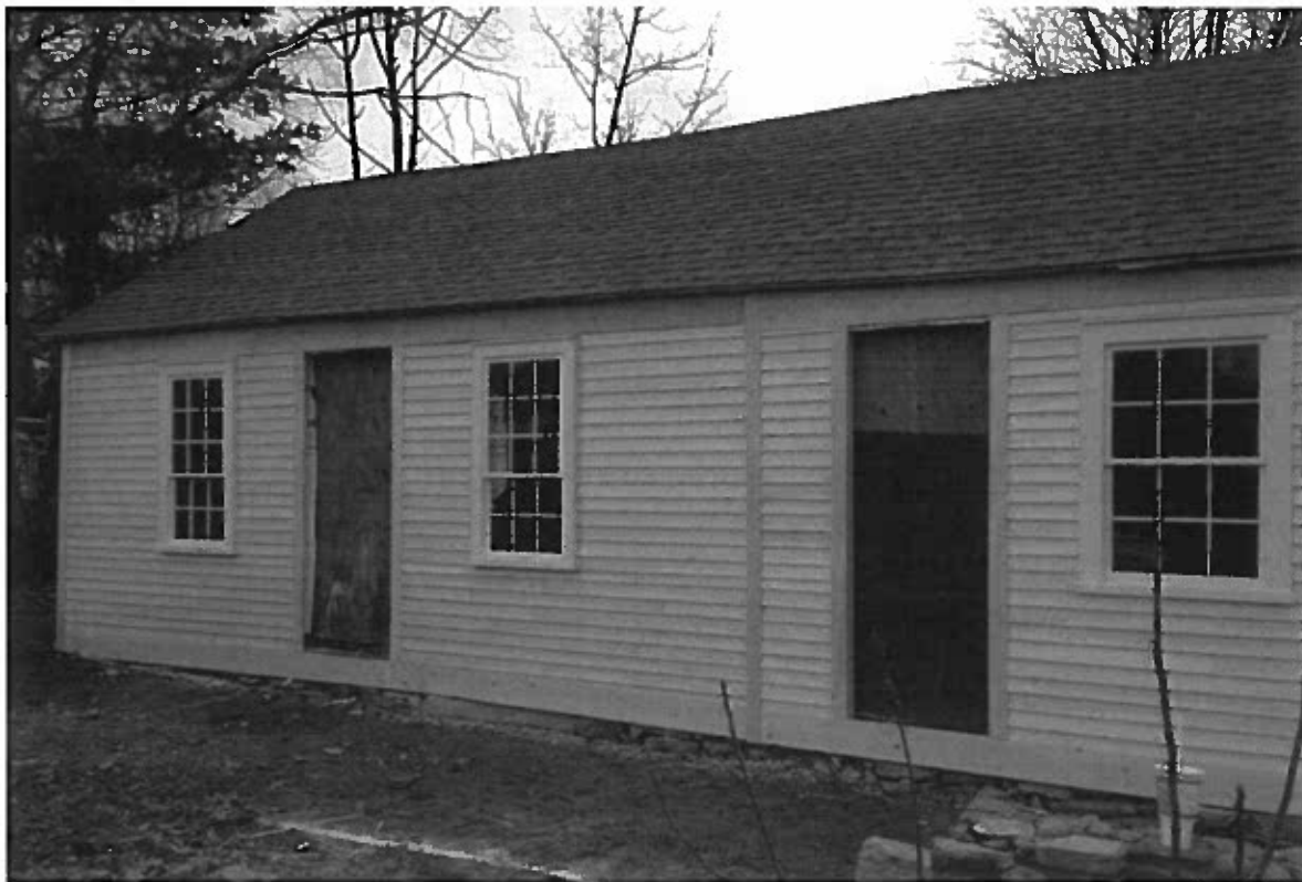
The façade of the Homestead during restoration of the exterior in Summer 2014 (top) and one year later (bottom). Stosz Construction completed restoration of three sides of the Homestead. Removal of the original sheathing revealed structural damage (see lower left corner as one example) requiring additional work not included in the original bid (a change order).
